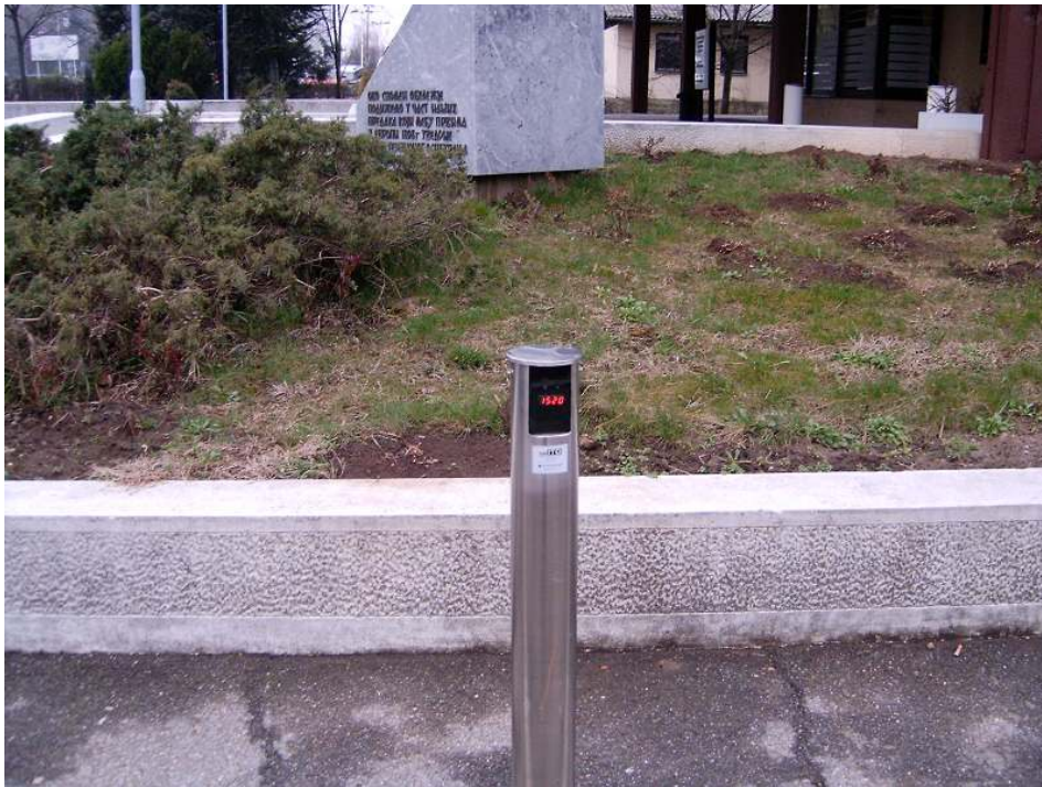
Fig.2 External antenna ITGant-6 (access control to parking lot)
